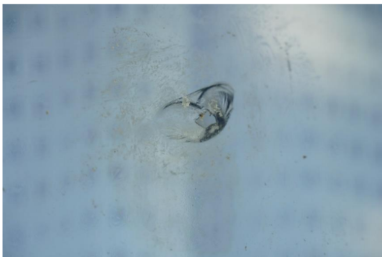
A hole of about 1 cm in diameter in a double-glazing window made of tempered glass
